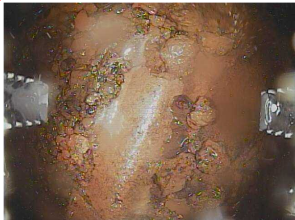
Before touching deposits
